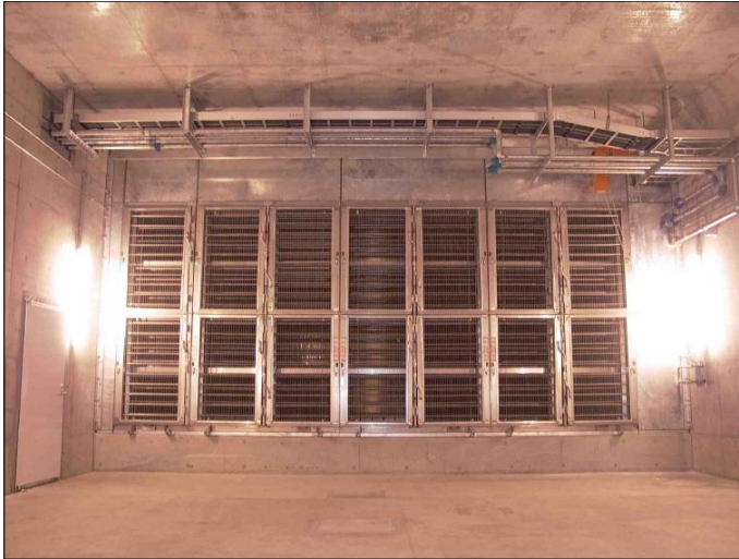
Fig 7. ESPs in a ventilation station
